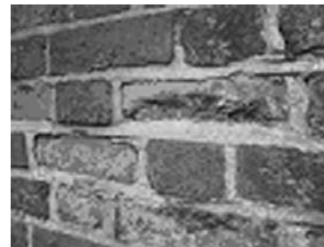
Hard cement pointing destroys soft bricks
