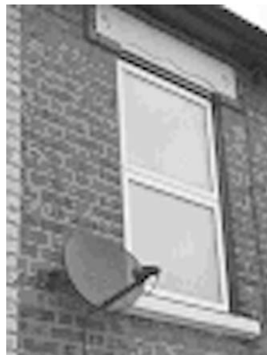
Unsympathetic replacement window and poorly sited satellite dish.
