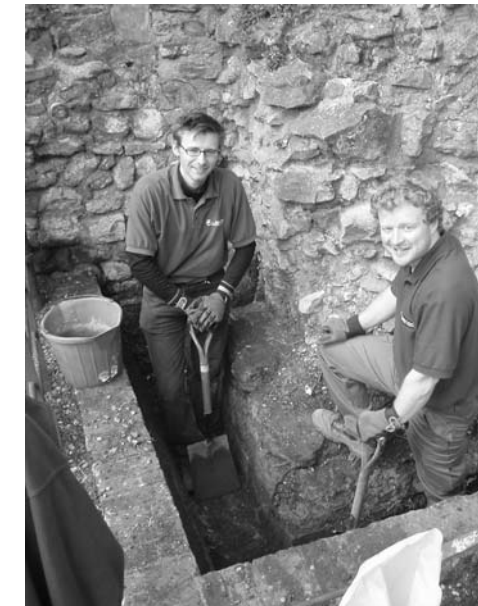
Jordan and Andy from Countrycare dig out 30 years of rubbish to once again reveal the only remaining part of the church existing above ground.
