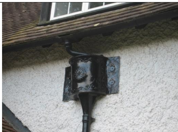
A cast iron gutter – an example of good practice
